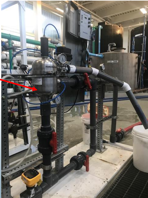
Sand Separator pilot skid
