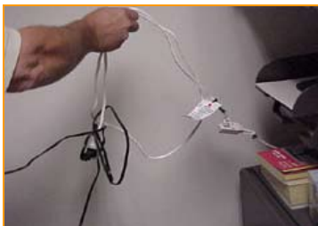
Use of non-approved multi-plug adaptors. (No Breaker)
