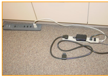
Power strip plugged into another power strip.
